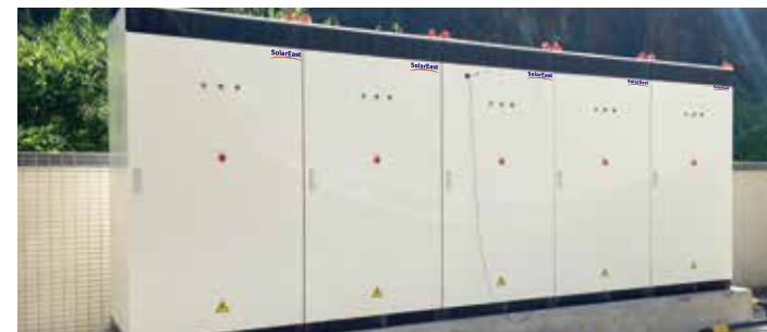
Industrial & Commercial Energy Storage Project, Guangdong
