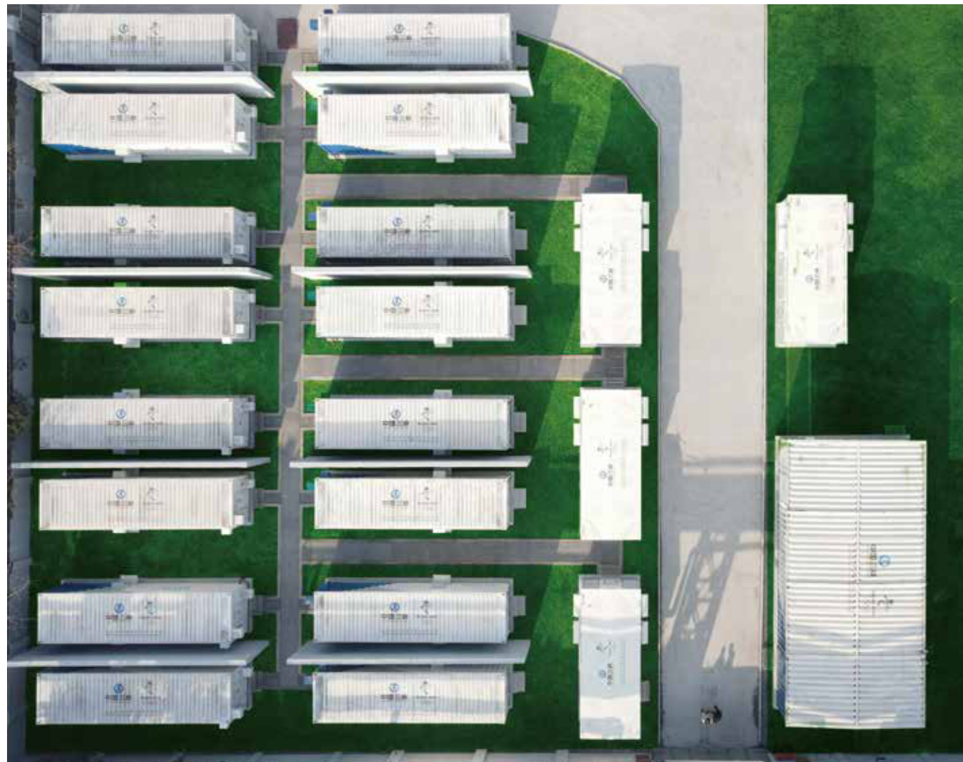
10MW/39MWh Energy Storage Station
